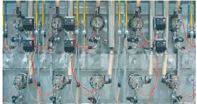
Roller hearth furnace
