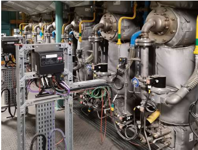
UNI-RAD system with plug-in-recuperator in a W-shaped radiant tube on a strip galvanising line
